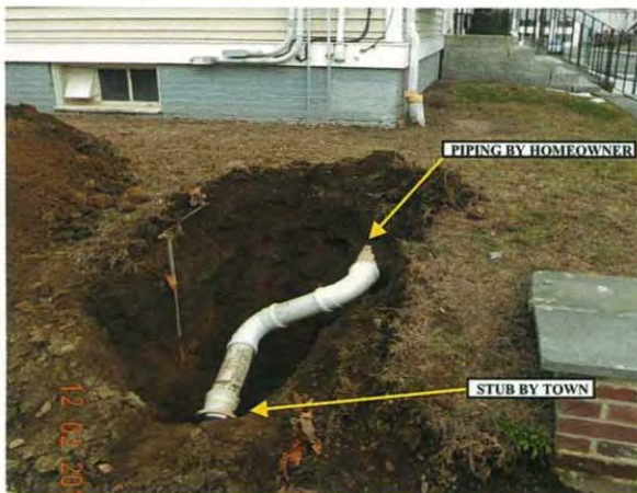
MUNICIPAL DRAIN SERVICES
