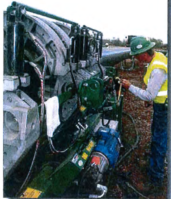
Quality control was a top priority for SAWS and ISCO. An ISCO field fusion technician logs information using a McElroy DataLogger™. The pipe is 24-inch DR 9.
