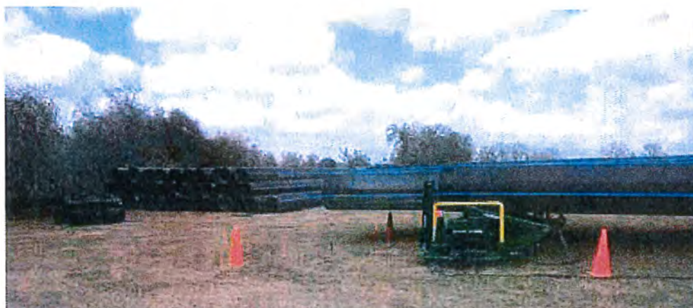
Staging of the pipe was imperative in a project as large as this one. Although this only shows a small portion of the pipe used, the ISCO team was highly organized to move large quantities of pipe as efficiently as possible.
