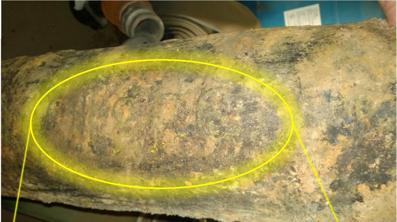
Winter Street water main circa 1886
