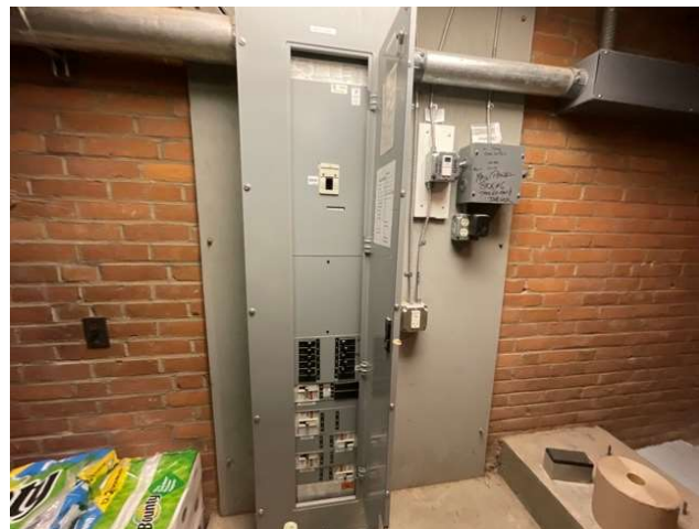
18 - MAIN SWITCH BOARD
