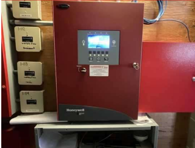
19 - FIRE ALARM SYSTEM
