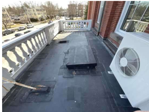
16 - DUCTLESS MINISPLIT CONDENSER
