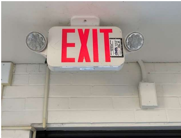
21 - EXIT SIGN WITH LIGHT
