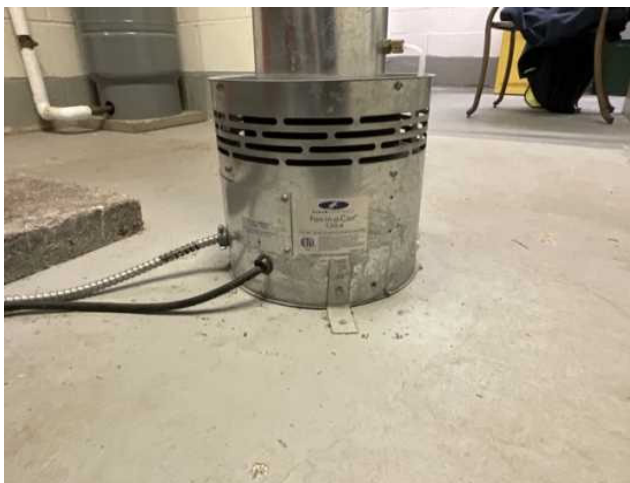
17 - MAKE-UP AIR BOILER ROOM
