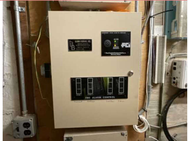
20 - FIRE ALARM SYSTEM
