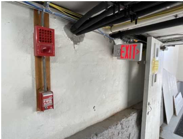
21 - FIRE ALARM DEVICES
