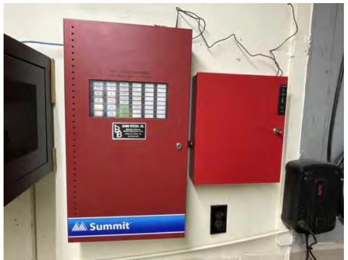
30 - FIRE ALARM PANEL
