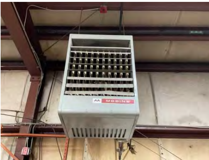
23 - UNIT HEATER THROUGHOUT GARAGES
