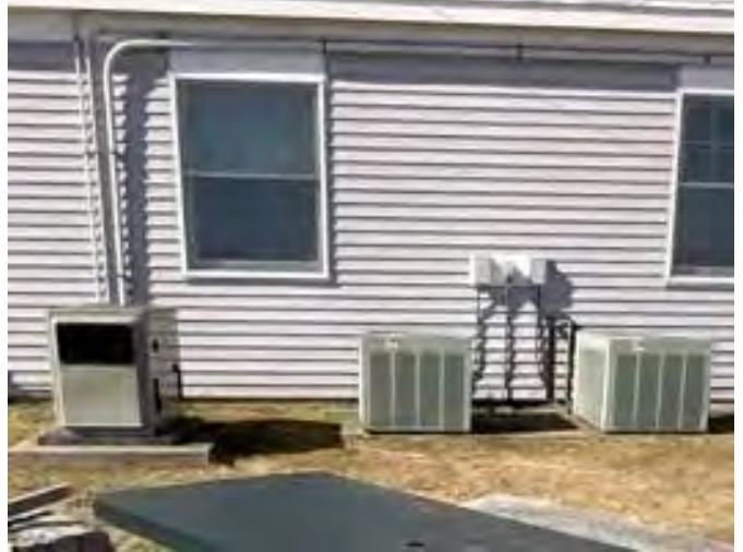
20 - CONDENSERS AND GENERATOR
