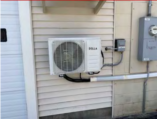
37 - SPLIT SYSTEM DUCTLESS
