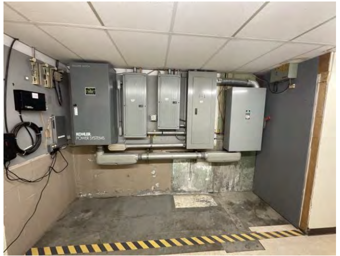
28 - MAIN ELECTRIC ROOM
