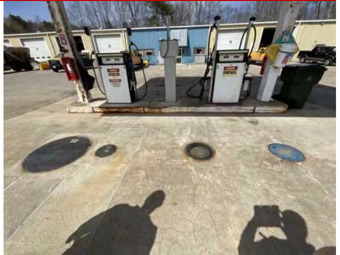
50 - STORAGE TANK, FUEL, 5001 TO 10000 GAL,
