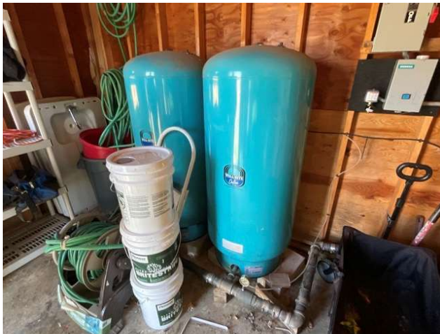
21 - STORAGE TANKS PUMPHOUSE
