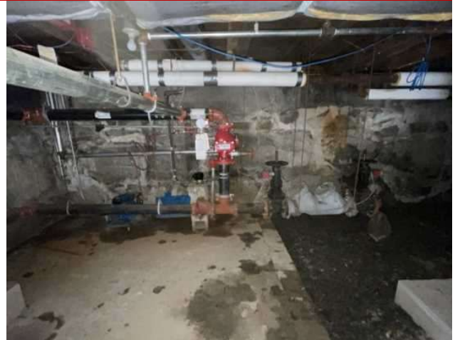
14 - FIRE SUPPRESSION SYSTEM
