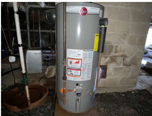
11 - HOT WATER TANK
