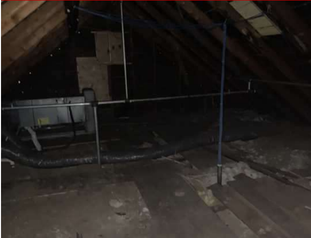
13 - ATTIC AIR HANDLER
