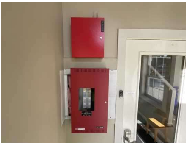
17 - FIRE ALARM SYSTEM
