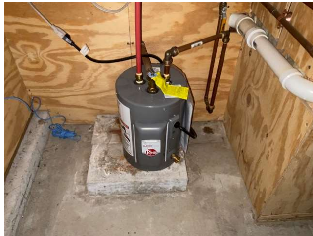
22 - SMALL DHW STORAGE SHED
