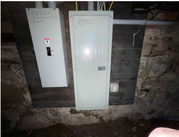
15 - MAIN ELECTRIC CRAWLSPACE
