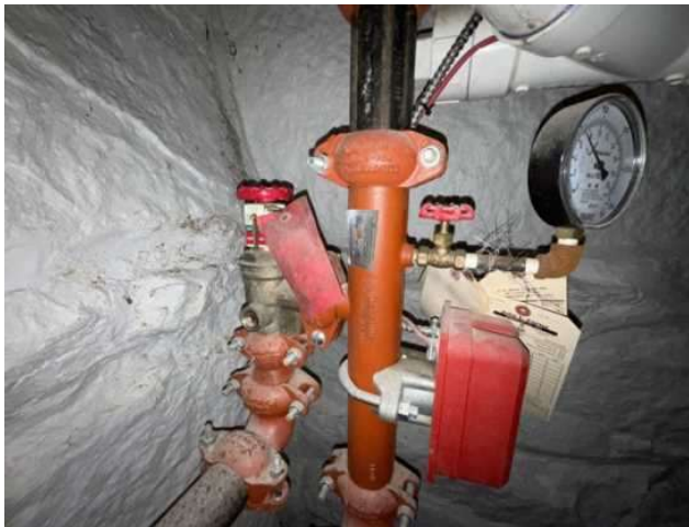
15 - FIRE SUPPRESSION SYSTEM
