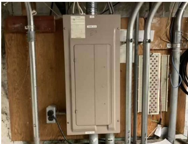
17 - MAIN ELECTRIC PANEL
