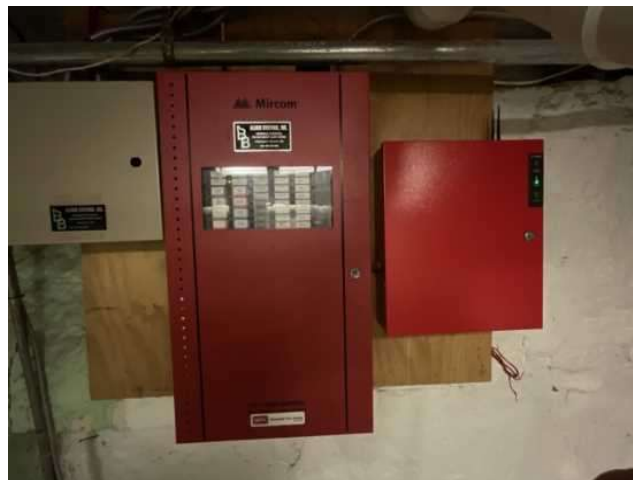
18 - FIRE ALARM SYSTEM
