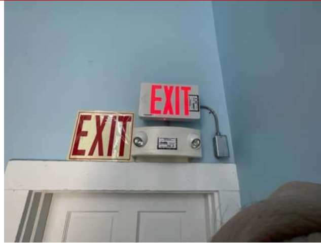
20 - EMERGENCY AND EXIT LIGHTING
