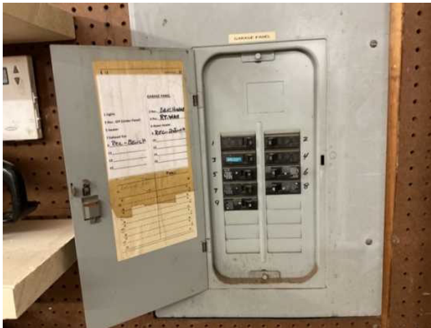
15 - MAIN ELECTRIC PANEL
