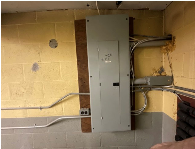
13 - MAIN ELECTRICAL PANEL
