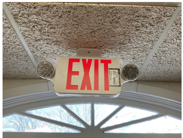
18 - EXIT SIGN WITH LIGHTING
