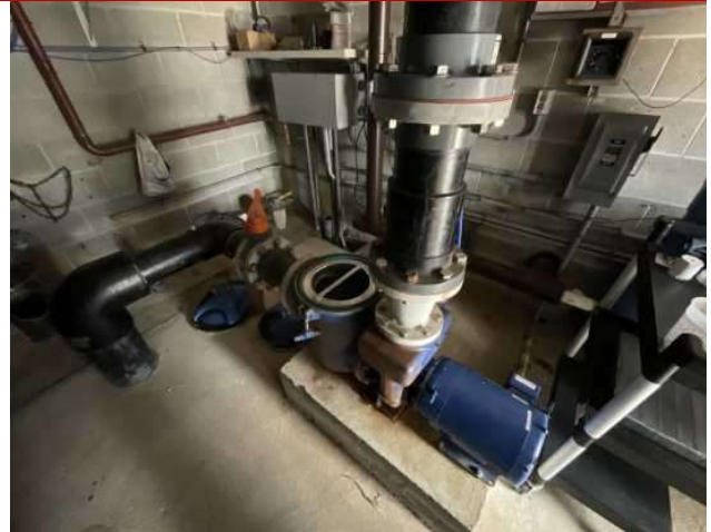
14 - POOL PUMP ROOM
