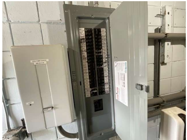
10 - MAIN ELECTRIC PANEL
