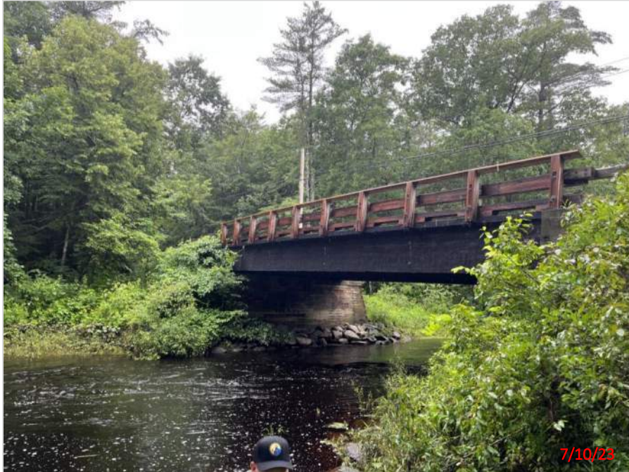
Photograph 1 – View of Linden Street Bridge South Abutment over Exeter River (Facing Southwest)
