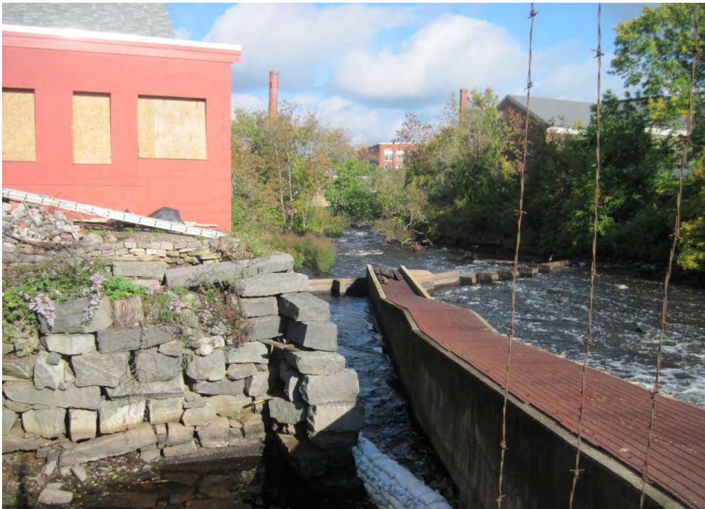
A. Left bank downstream of Great Dam. Rock retaining walls that appear to be sliding and have recently been stabilized.
