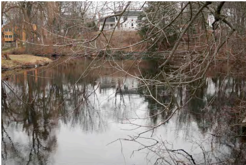
B. Sharp right angle bend in the Exeter River upstream of the dam may be prone to increased erosion after dam removal. Note: This photo location is shown as Area of Concern 1 labeled in Figure 3.3-1.
