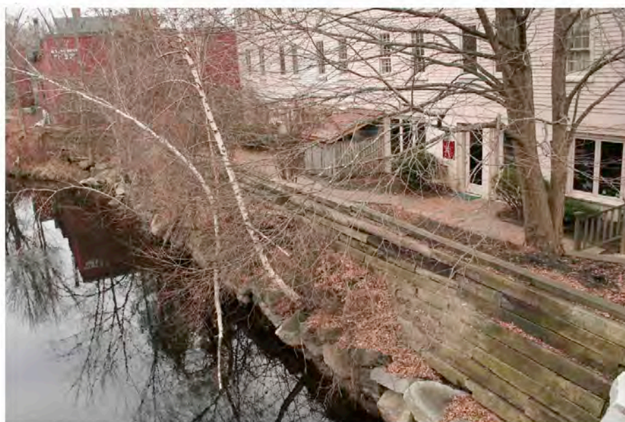
B. Upstream of Great Bridge – The banks are protected by a) rock walls and b) retaining walls
