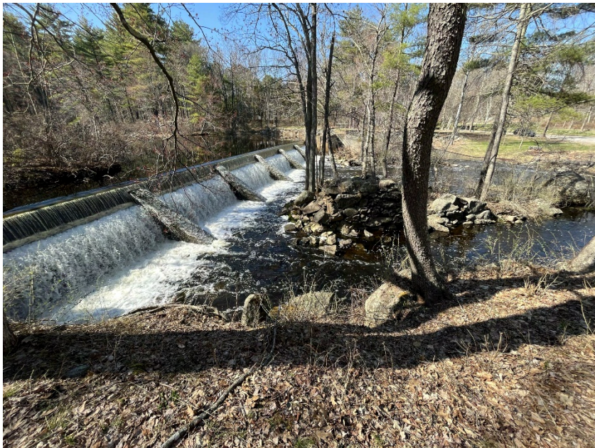
An oblique view of Pickpocket Dam primary spillway, looking from the right bank
