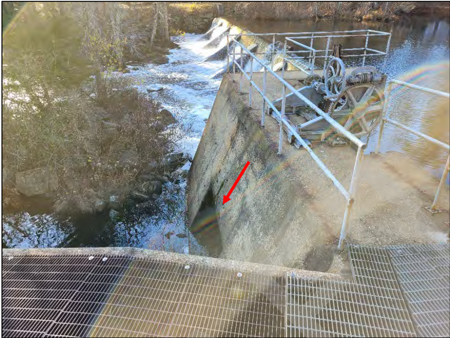
Photo No. 7.: Overview of the downstream side of the low-level outlet discharge (arrow) and the spillway.
