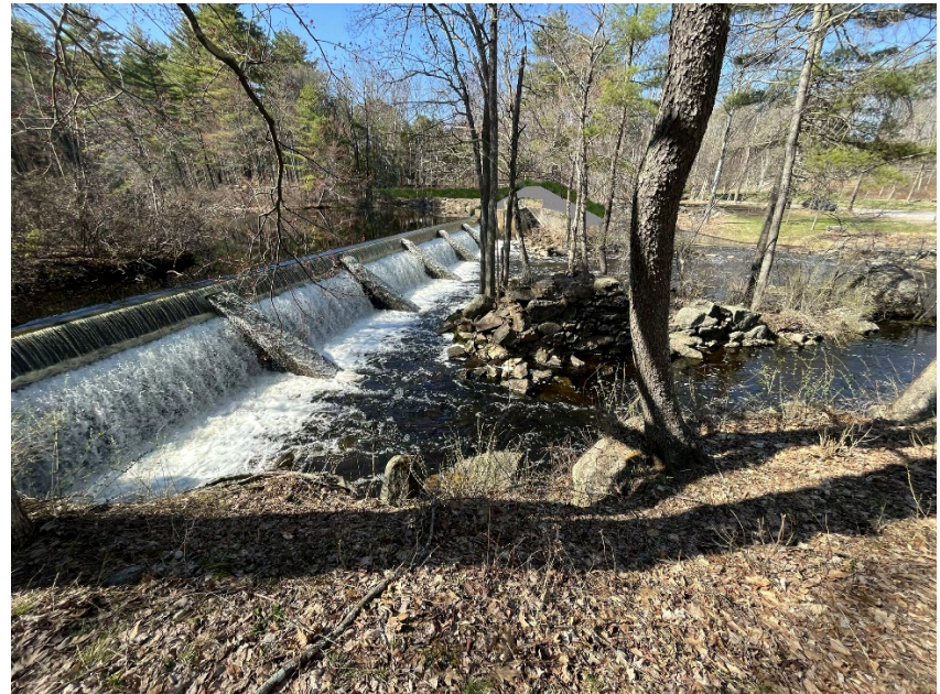
An oblique view of Pickpocket Dam primary spillway with Alternative 1, looking from the right bank
