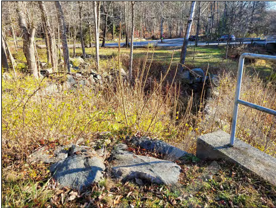
Photo No. 11.: Downstream slope from the edge of left training wall. Note the vegetation growth within the rip rap and abandoned stone foundation.
