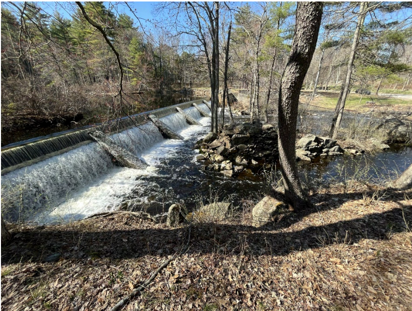
An oblique view of Pickpocket Dam primary spillway, looking from the right bank
