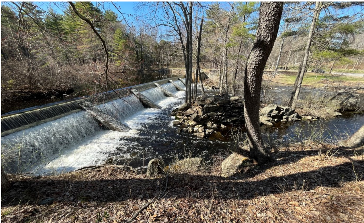
Side view of Pickpocket Dam and spillway looking north, from right bank
