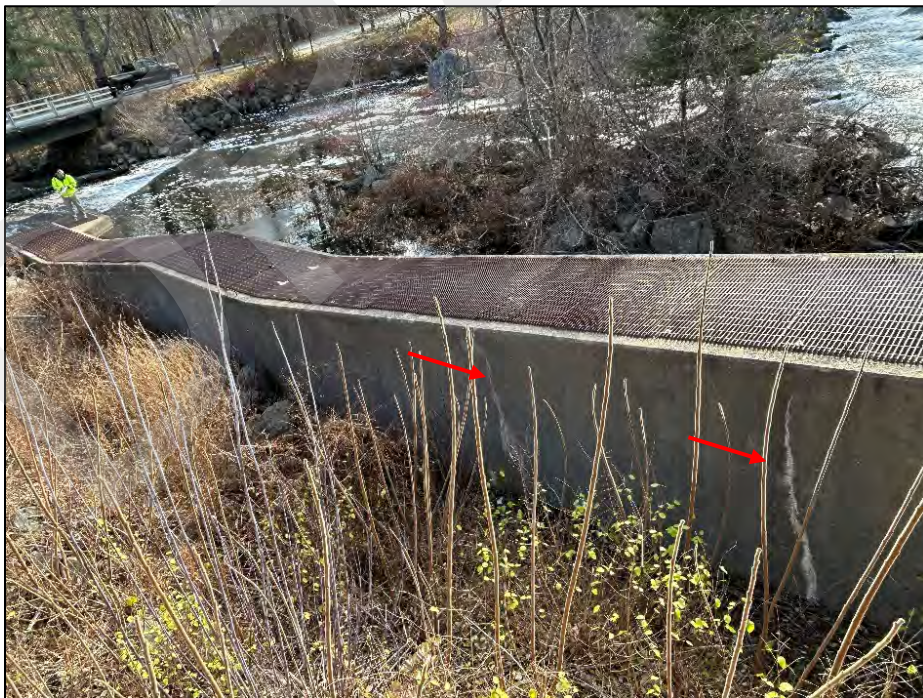
Photo No. 22.: Fish ladder looking downstream from left training wall of the spillway. Note cracks (arrows) with efflorescent staining along the walls.
