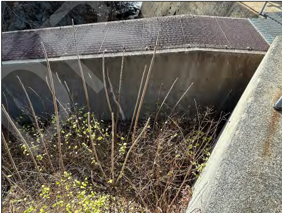
Photo No. 20.: Upstream portion of the concrete fish ladder from the left downstream training wall.
