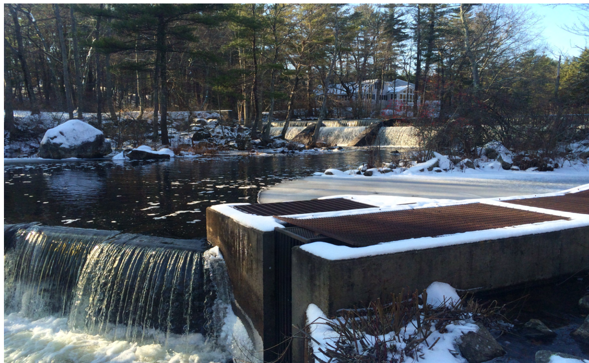
View of the fish ladder downstream of Pickpocket Dam at training weir.
