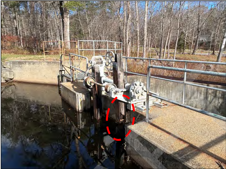
Photo No. 17.: View of the low-level outlet operator/approach. The gate is inoperable due to deteriorated timber stems (circled).
