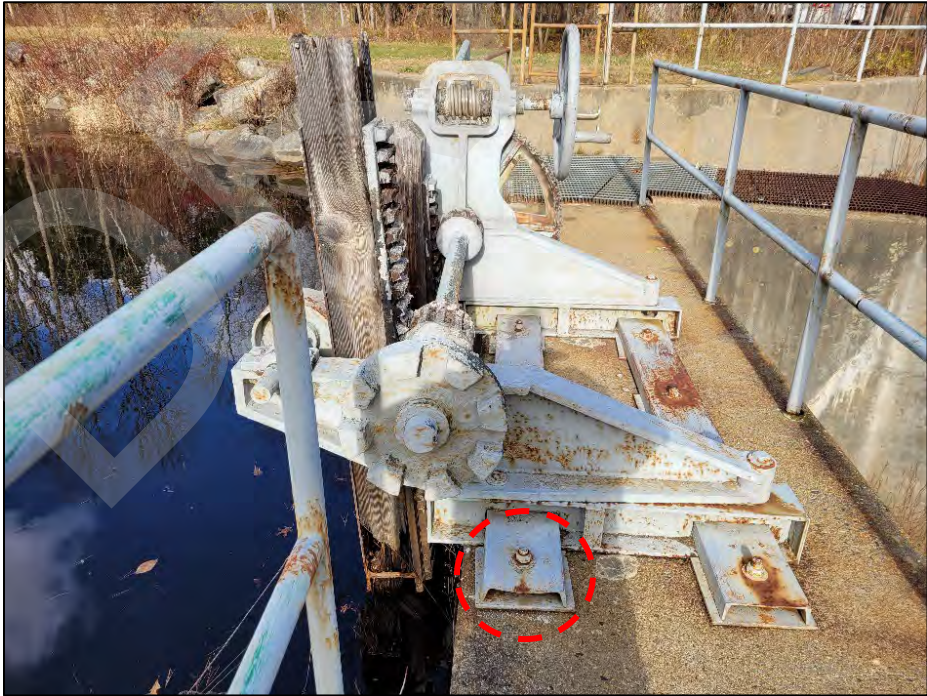
Photo No. 18.: A bent channel support (circled) for the low-level outlet gate and gears for the stems are corroded.
