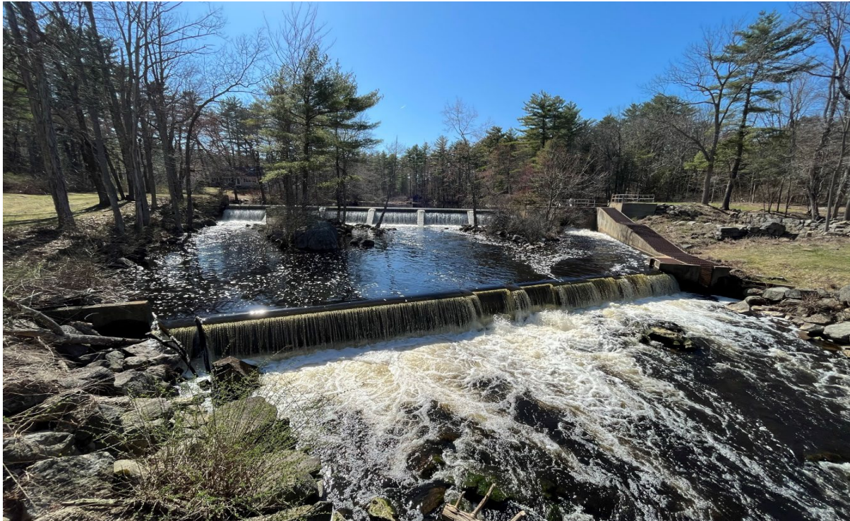
High-level view of Pickpocket Dam looking upstream from right bank at Cross Road
