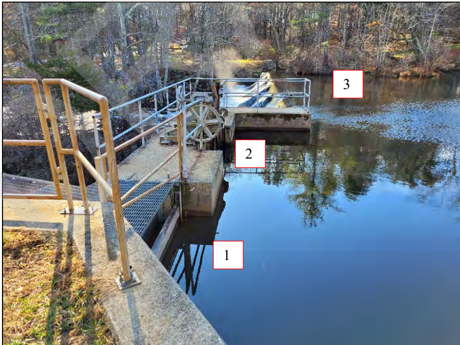
Photo No. 2.: Overview of the fishway entrance (1), low-level outlet entrance (2), and primary spillway (3) from the left training wall.
