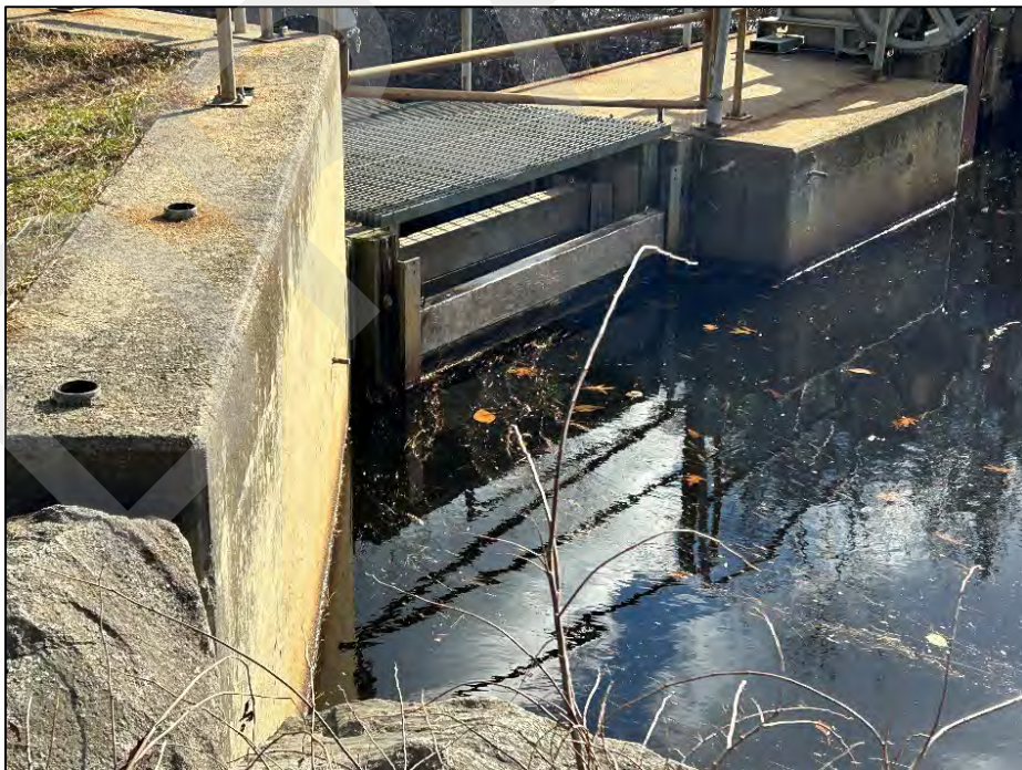
Photo No. 16.: Upstream stoplogs and stoplog slots for fish ladder. Stoplogs are fitted with lifting hooks for removal.
