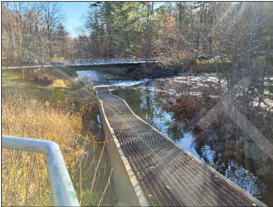
Photo No. 5.: Minor leakage between the left downstream slope and fish ladder.
