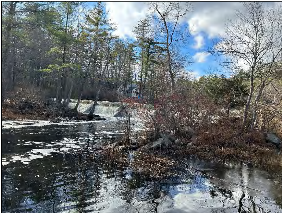
Photo No. 14.: Downstream discharge area for the low-level outlet and primary spillway from the end of the fish ladder.
