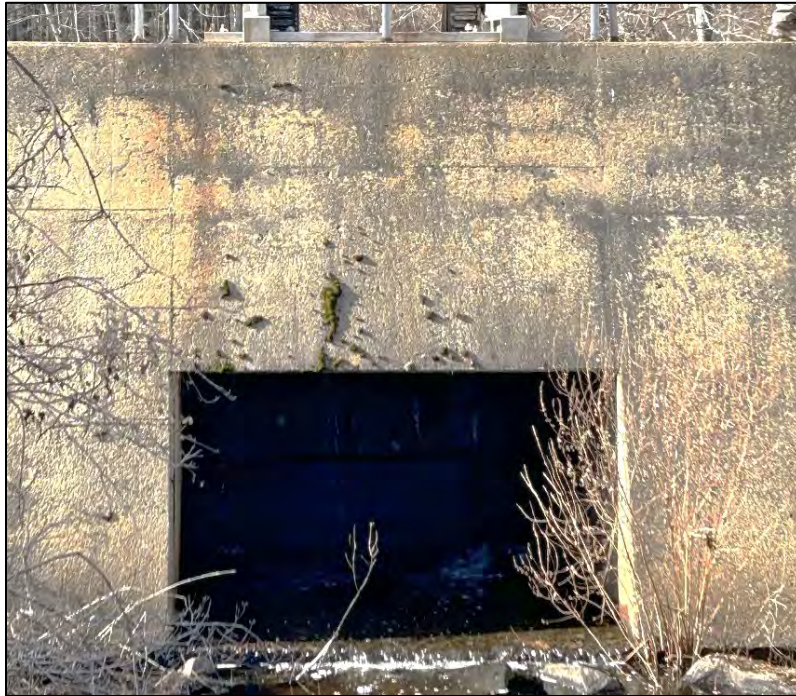
Photo No. 19.: Discharge for the low-level outlet from downstream channel. The gate is leaking from the left side of the structure.
