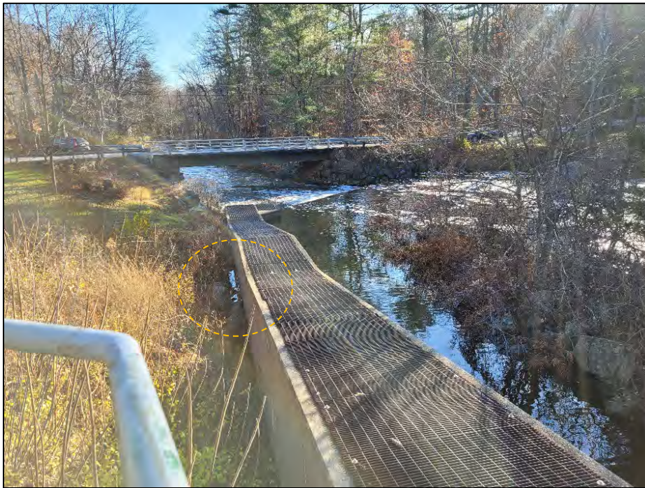
Photo No. 5.: Minor leakage between the left downstream slope and fish ladder.
