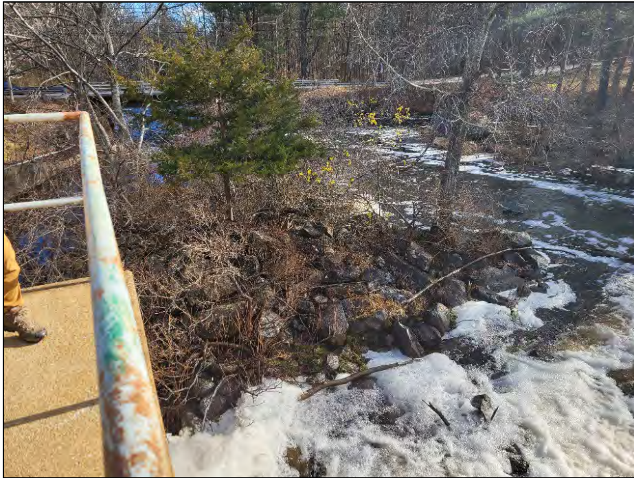
Photo No. 13.: Downstream stone and vegetation area between LLO and spillway crest.
