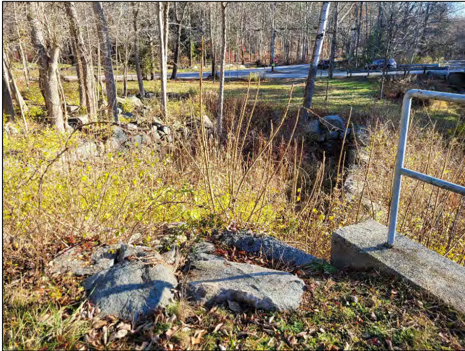
Photo No. 11.: Downstream slope from the edge of left training wall. Note the vegetation growth within the rip rap and abandoned stone foundation.
