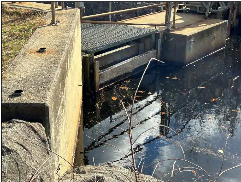
Photo No. 16.: Upstream stoplogs and stoplog slots for fish ladder. Stoplogs are fitted with lifting hooks for removal.
