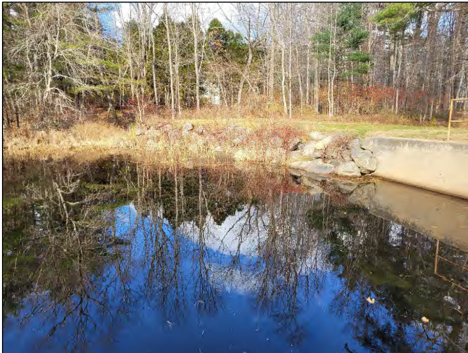
Photo No. 10.: Upstream riprap at left abutment/embankment. Note vegetation growth within the riprap on the slope at the abutment.
