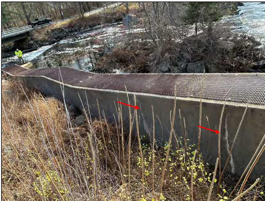
Photo No. 22.: Fish ladder looking downstream from left training wall of the spillway. Note cracks (arrows) with efflorescent staining along the walls.
