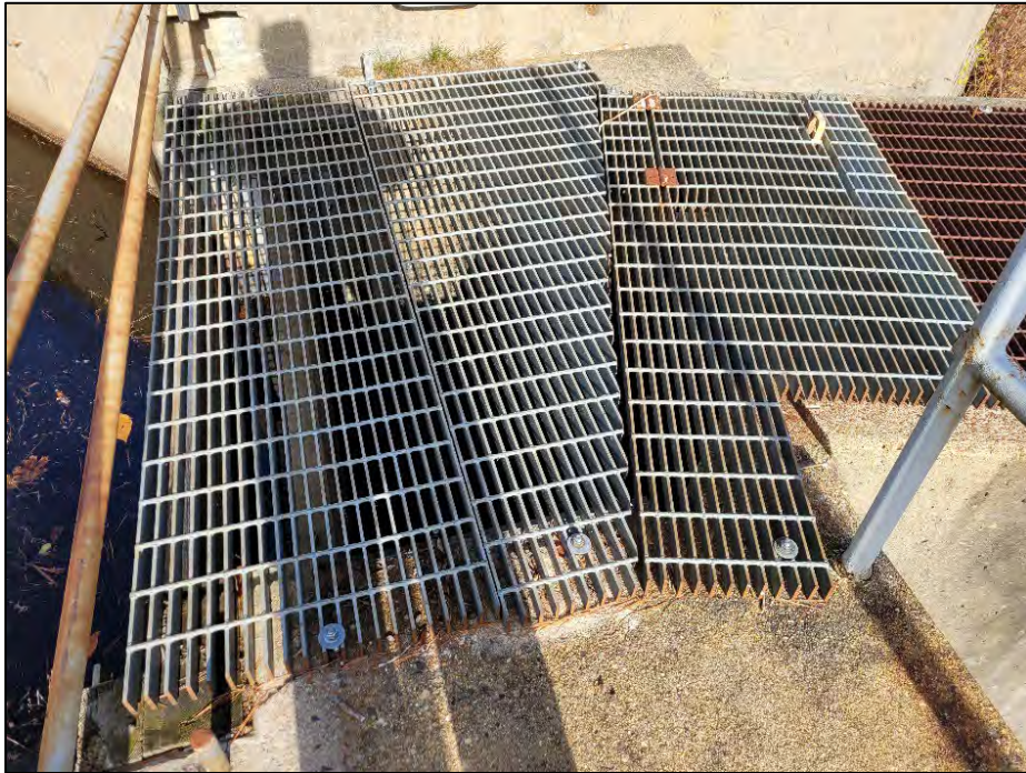
Photo No. 23.: Upstream stoplogs and stoplog slots for fish ladder. Stoplogs have lifting hooks for removal. Note steel grating must be removed to adjust stoplogs
