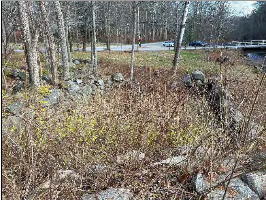
Photo No. 27.: The remnants of an old stone foundation left of the fishway. Wet areas inside the foundation were noted.
