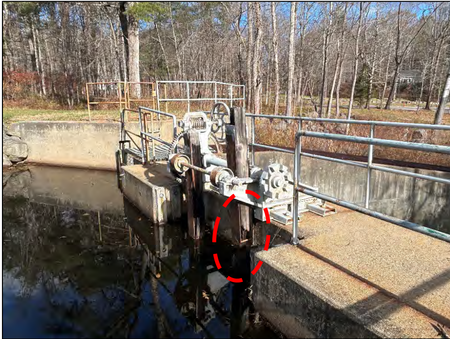
Photo No. 17.: View of the low-level outlet operator/approach. The gate is inoperable due to deteriorated timber stems (circled).
