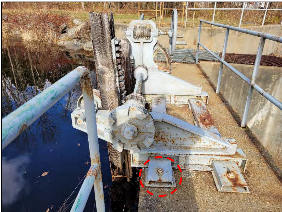
Photo No. 18.: A bent channel support (circled) for the low-level outlet gate and gears for the stems are corroded.
