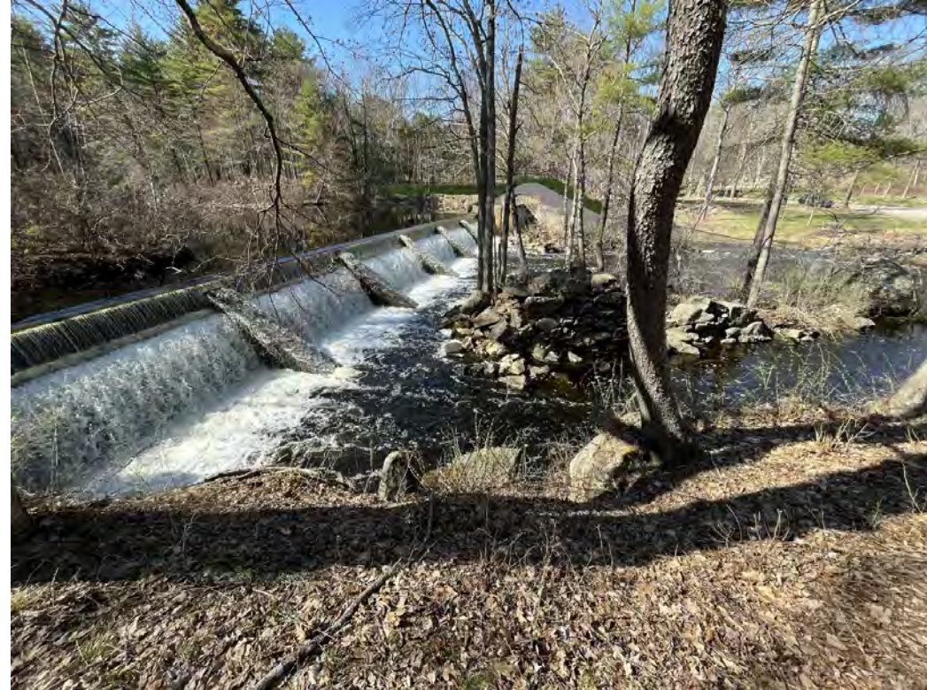
An Oblique view of Pickpocket Dam with Alternative 1, looking from the right bank
