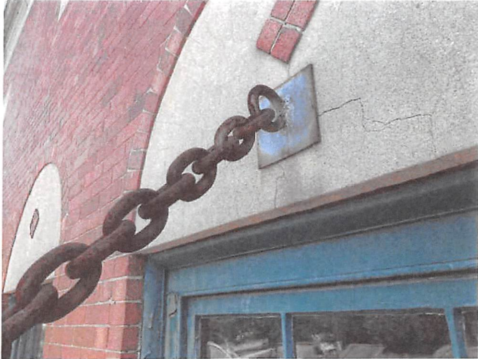
Photo #3 – Stress cracks at sign attachment to building
