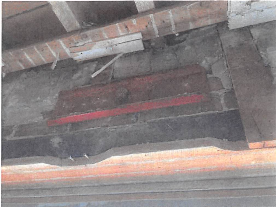
Photo #4 – Stress cracks on interior of sign attachment
