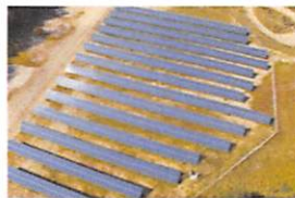
Town of Durham Sand Pit, Police Dept, Library, Ice Rink 780 kW (2014-16)
