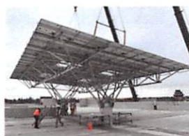
Manchester Langer Place Parking Garage (with SNHU); 1MW RFP award (2019)
