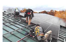
City of Nashua Transit Garage, Fire Station, Ice Arena 1.6 MW (2019-20)
