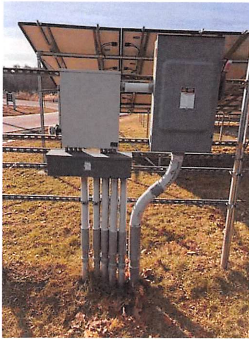
6.0 Conduit, Raceways, BOS - General photos
