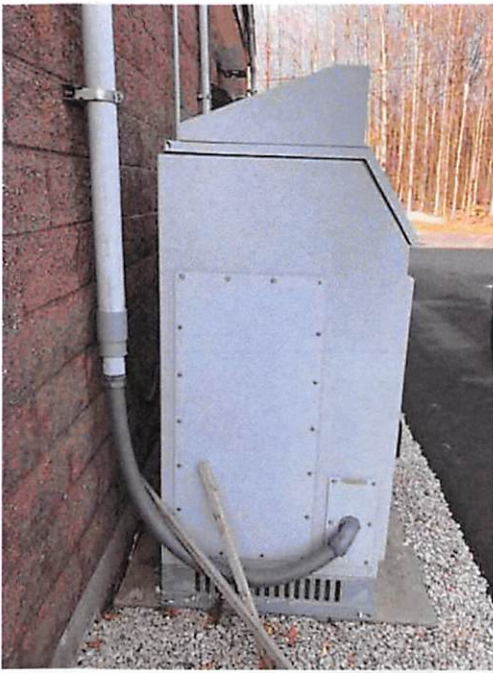
6.0 Conduit, Raceways, BOS - General photos
