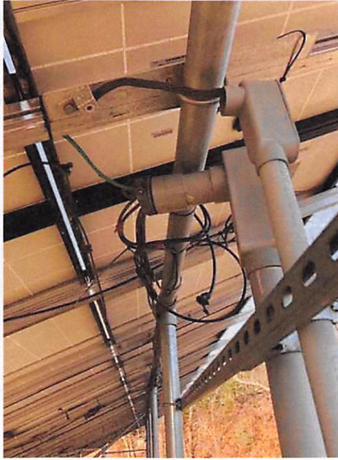
5.0 Modules and Racking - Wire management: secured, drip loops, metal ties
