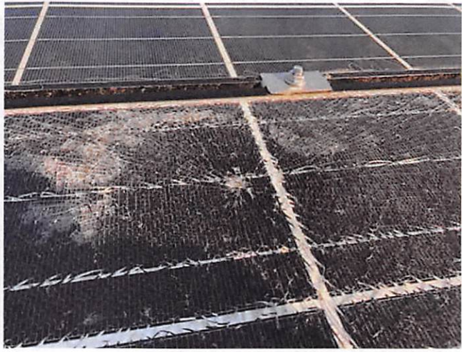
5.0 Modules and Racking - Modules: damage, delamination, discoloring
