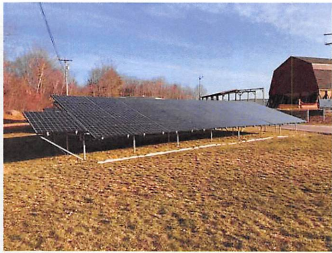
5.0 Modules and Racking - General photos
