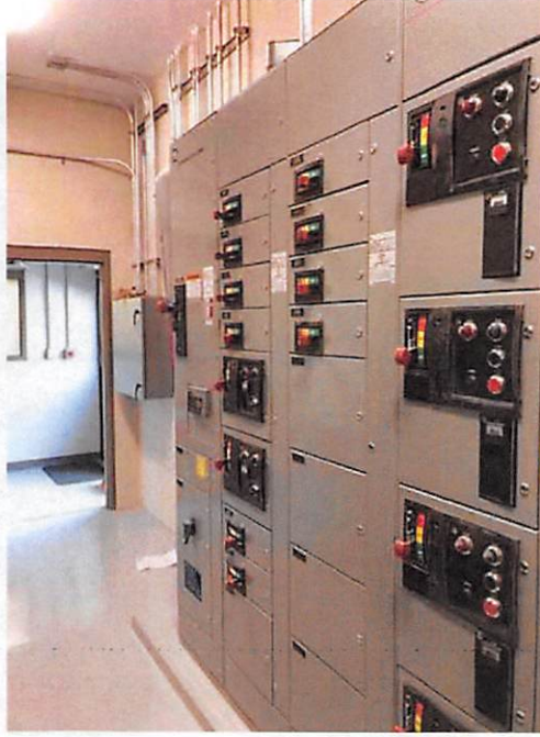
4.0 AC Components (meters, discos, switch gear, transformers) - General photos
