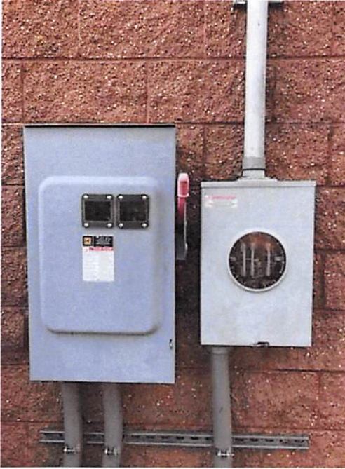
4.0 AC Components (meters, discos, switch gear, transformers) - Signage and labeling: legible, firmly attached
