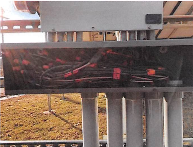
3.0 DC Components (discos, combiners, recombiners, etc.) - Conductors: routing and wire management, labeling/color coding, protected from damage
