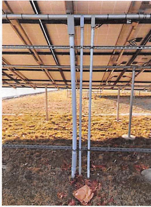
6.0 Conduit, Raceways, BOS - General photos
