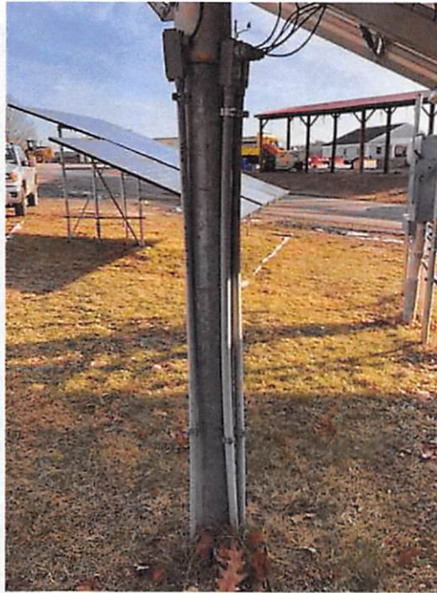
6.0 Conduit, Raceways, BOS - General photos
