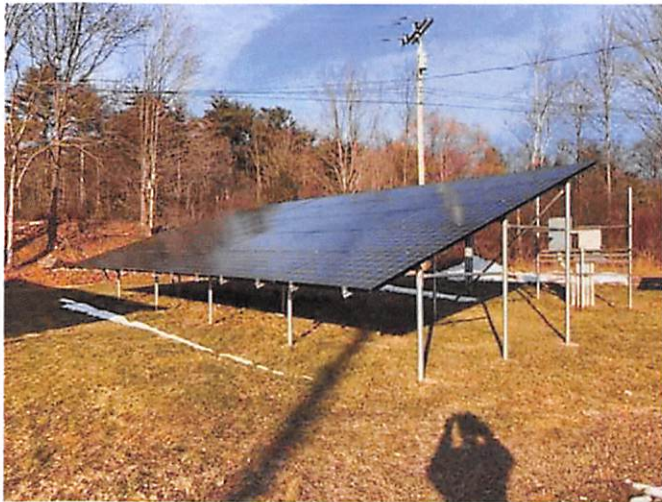
5.0 Modules and Racking - General photos
