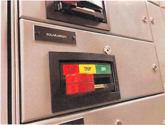
4.0 AC Components (meters, discos, switch gear, transformers) - General photos
