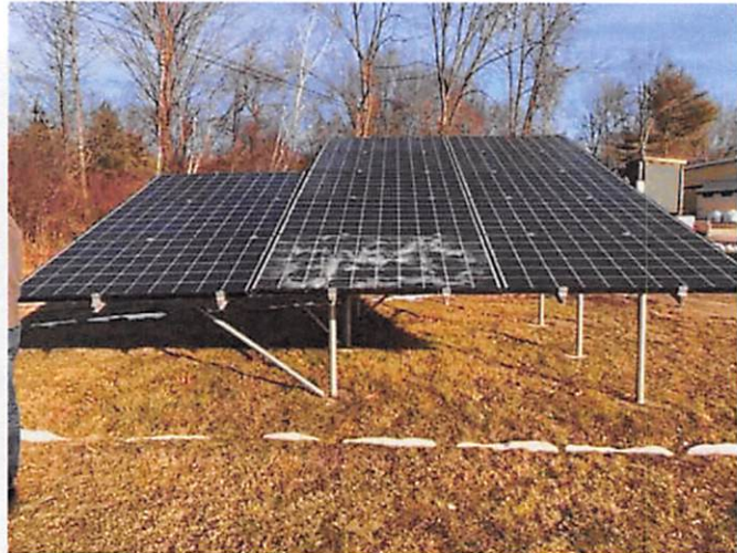
5.0 Modules and Racking - Modules: damage, delamination, discoloring
