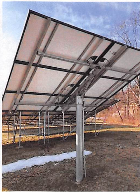
5.0 Modules and Racking - General photos
