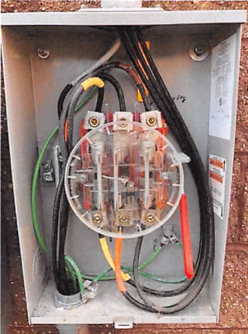
4.0 AC Components (meters, discos, switch gear, transformers) - Mounting and Enclosure condition: secure, clean and free of debris/dirt/moisture
