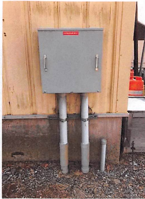
6.0 Conduit, Raceways, BOS - General photos
