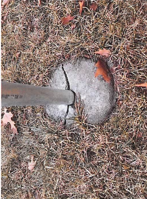
5.0 Modules and Racking - Structural integrity: damage, rust, row shifting (frost heave, ground movement)
