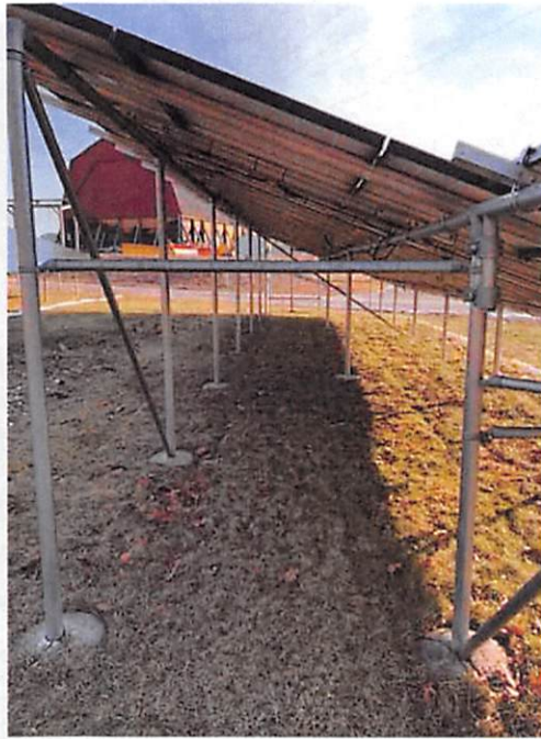
5.0 Modules and Racking - General photos
