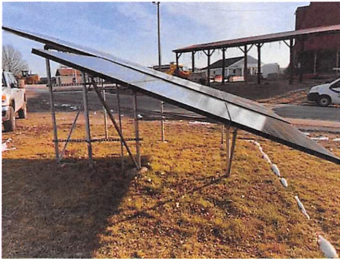
5.0 Modules and Racking - General photos
