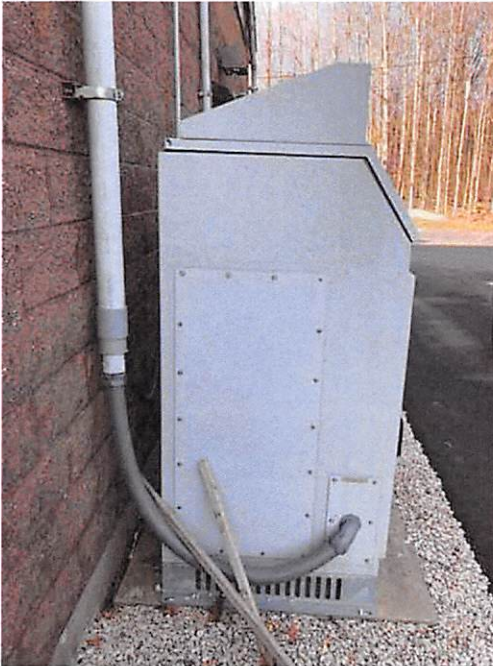
2.0 Inverters - Integrity of the enclosure: penetrations, supports, fittings, door hinges, interior/exterior clean and free of debris, no moisture or rust
