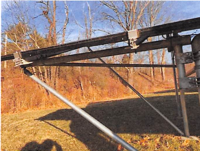
5.0 Modules and Racking - General photos
