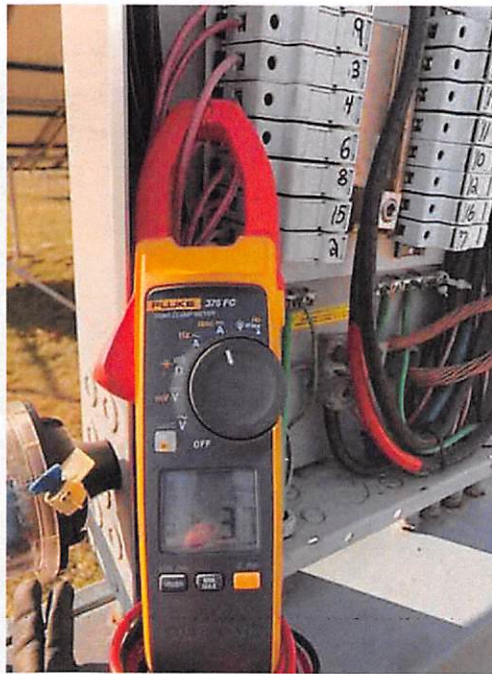
3.0 DC Components (discos, combiners, recombiners, etc.) - General photos
