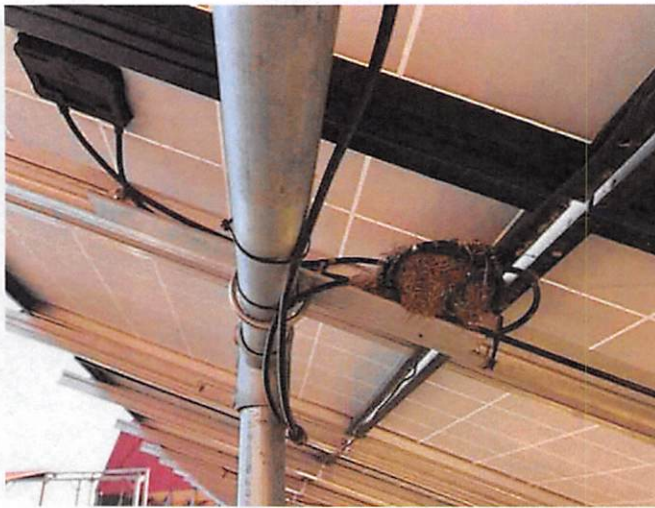
5.0 Modules and Racking - Wire management: secured, drip loops, metal ties
