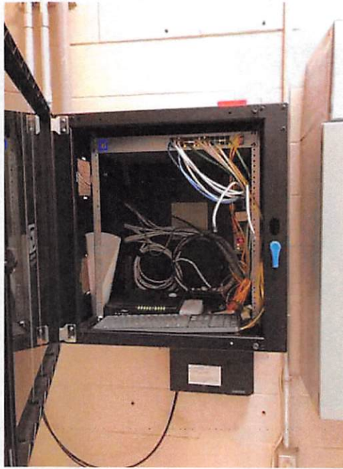
7.0 DAS/SCADA and Weather Station - General photos
