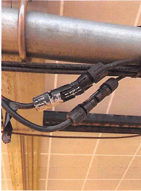
5.0 Modules and Racking - Leads, connectors, homeruns: damage, loose or failed connectors
