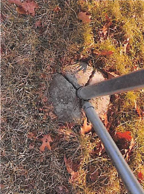
5.0 Modules and Racking - Structural integrity: damage, rust, row shifting (frost heave, ground movement)
