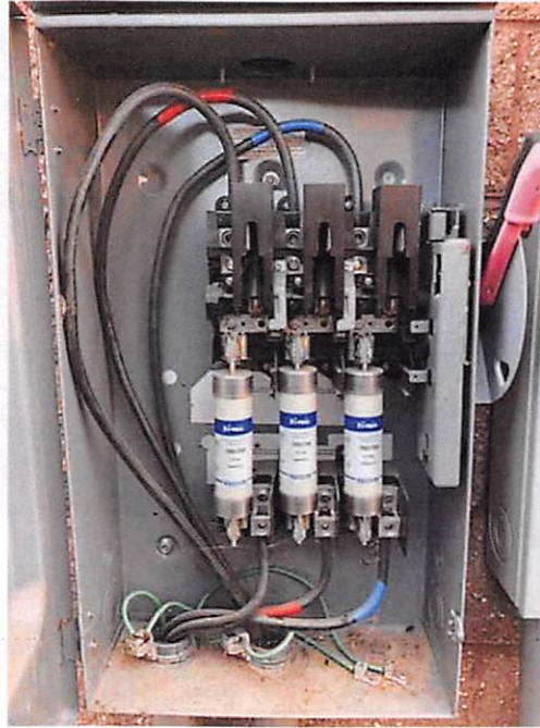
4.0 AC Components (meters, discos, switch gear, transformers) - Mounting and Enclosure condition: secure, clean and free of debris/dirt/moisture
