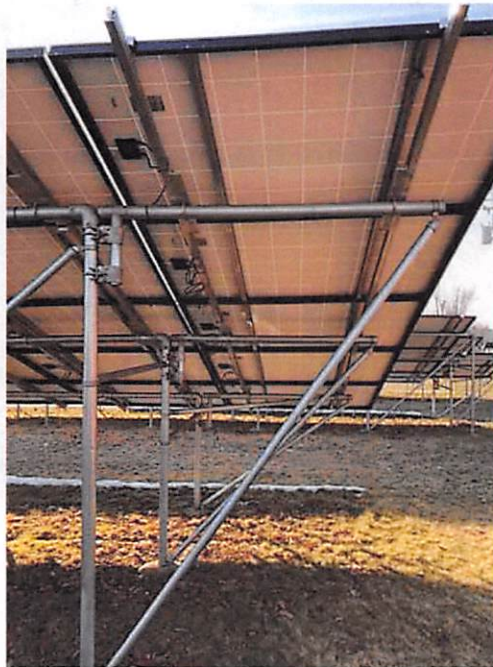
5.0 Modules and Racking - General photos
