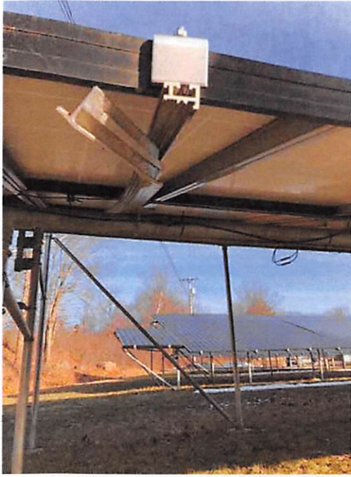
5.0 Modules and Racking - Structural integrity: damage, rust, row shifting (frost heave, ground movement)
