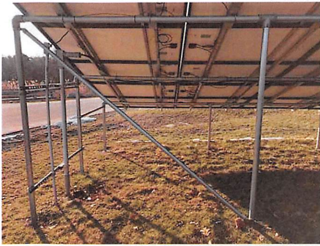
5.0 Modules and Racking - General photos
