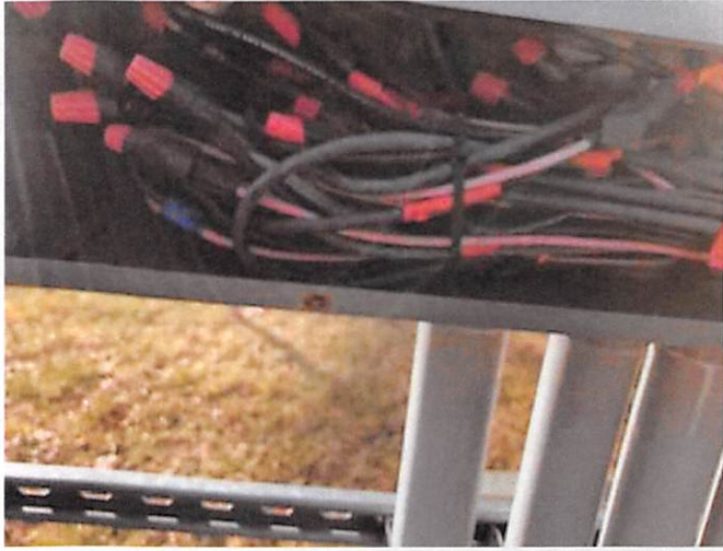
3.0 DC Components (discos, combiners, recombiners, etc.) - Conductors: routing and wire management, labeling/color coding, protected from damage
