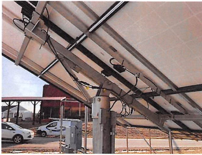
5.0 Modules and Racking - General photos
