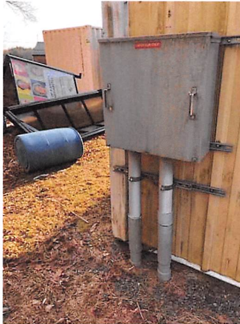
6.0 Conduit, Raceways, BOS - General photos
