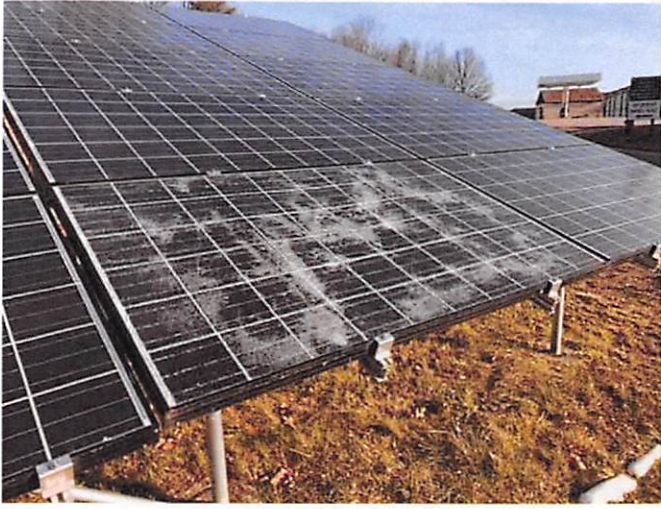
5.0 Modules and Racking - Modules: damage, delamination, discoloring
