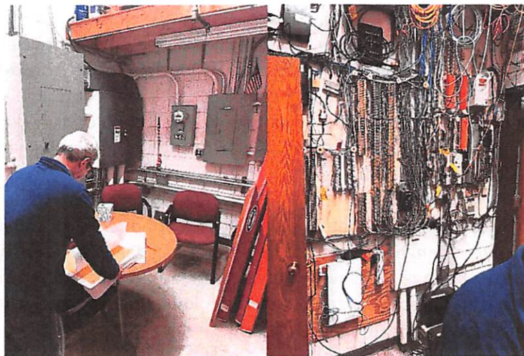
So-called Interview Room Adjacent to Front Lobby Access to exposed wiring presents several hazard/risk factors.
