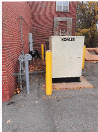
Figure 16 – Unsecured utilities and backup generator
