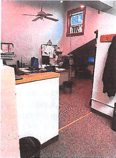
Detective Workspace Re-purposed from lobby atrium Floors uneven Roof leaks
