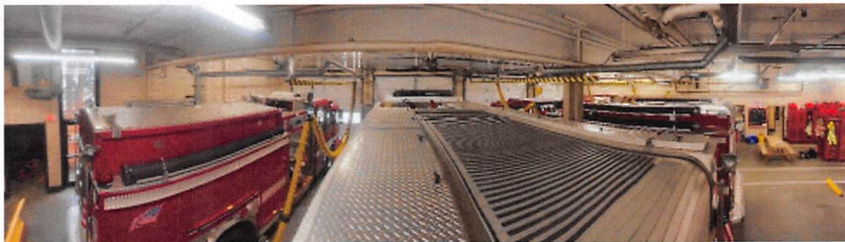
Figure 910– Lack of Clearance – Operational Inefficiency - Low ceiling height prevents easy hose loading or filling engines with water.
