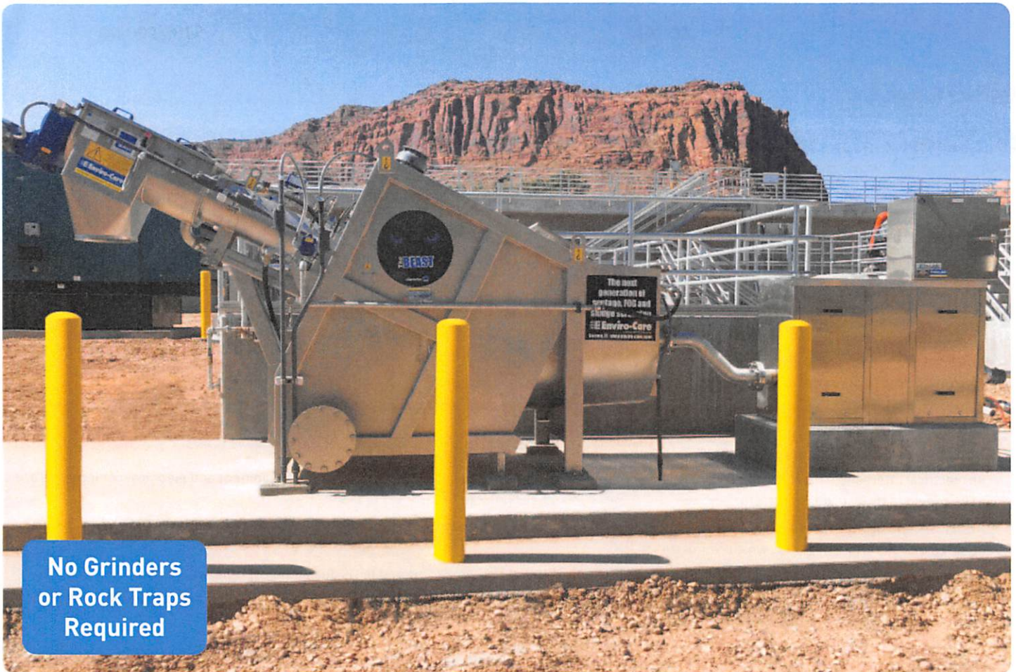
Septage BEAST Property of Moab UT
