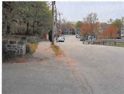
Deficient sidewalk and crossing at Chestnut Street and Woodlawn Circle.
