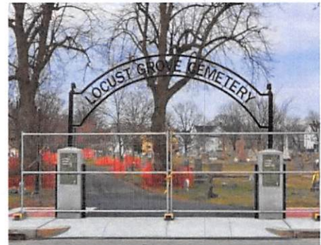
Top: Graphic illustration of designed cemetery entrance. Bottom: Construction photo, Locust Grove Cemetery Entrance Improvements, Providence Park Dept - Ironwood 2023
