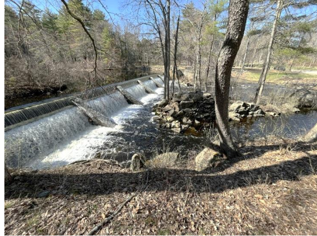
An oblique current view of Pickpocket Dam primary spillway, looking from the right bank
